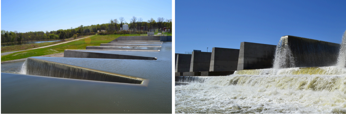
Fig. 13. Staged labyrinth spillway at Lake Townsend, Greensboro, NC, USA (Photo taken by Brian Crookston)
